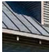
Metal Roof Accents
