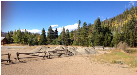
Base course removed from the medians and delivered to the Ice Arena
