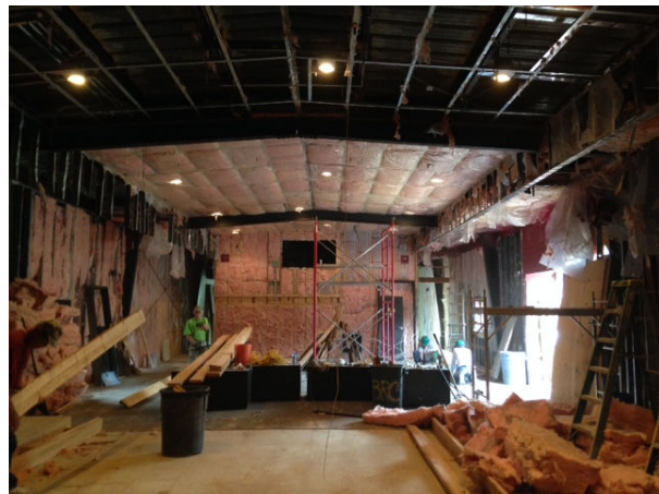
View into the simplistic 1960's steel Butler Building from the existing stage. The seating, risers, ceilings, and wall finished have been removed.
