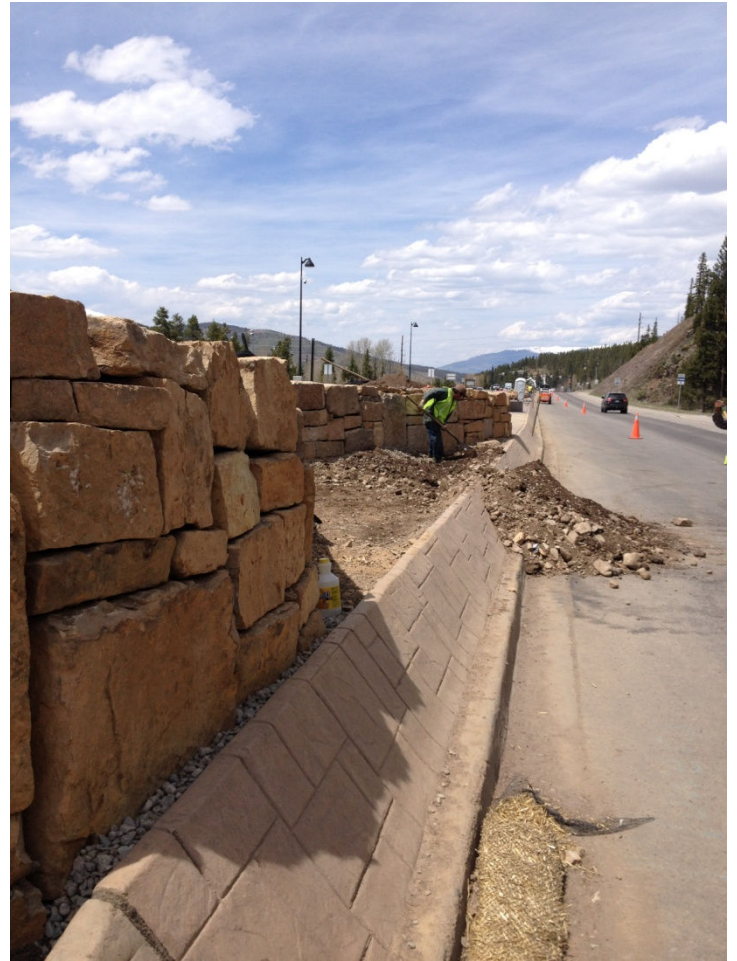
Stone retaining walls being constructed in the medians north of the roundabout.
