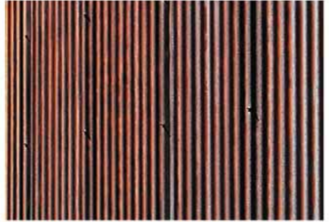
CORRUGATED RUSTED METAL SIDING
