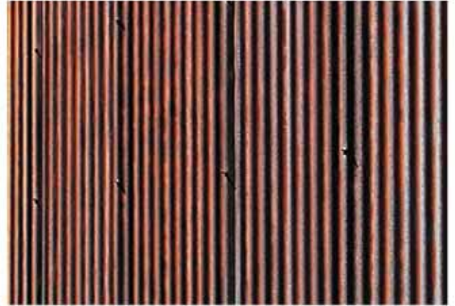
CORRUGATED RUSTED METAL SIDING
