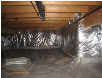
Crawl space conversion, insulation, radiant barrier and vapor barrier. Reduced air leakage, moisture infiltration and improved comfort in living space above.
