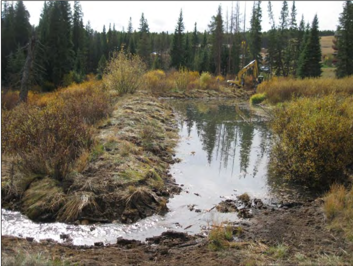
Photo C1a. The outlet spillway of the northern cell of the spreader pond in 2012 immediately after construction.
