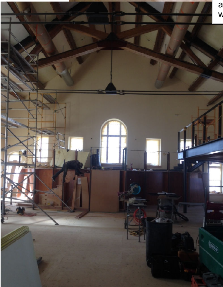
Work is continuing on the installation of millwork and stairs and 1021 buildings.
