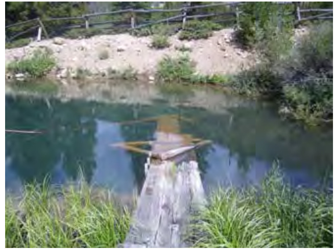
Fallen superstructure visible underwater.
