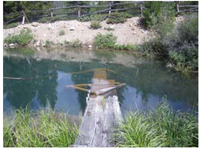
Fallen superstructure visible underwater.
