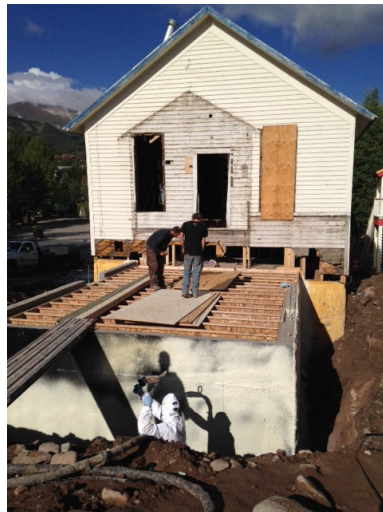
Insulation is applied to the foundation walls and framing started for the new addition.
