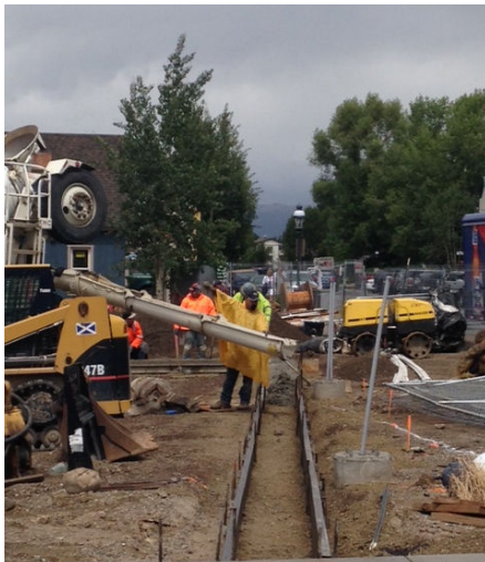
Concrete crews finish pouring curb in the new parking area as the afternoon showers begin.
