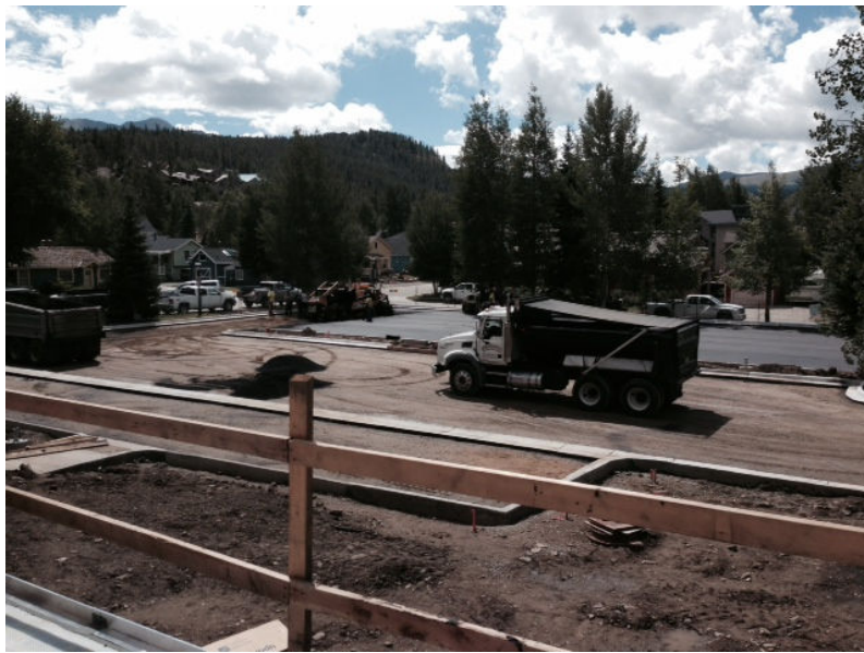
Left: Sunny weather allows the contractor to begin with paving of the south parking lot. The lot has been regraded to provide proper drainage and an ADA parking spot was added near the building.
