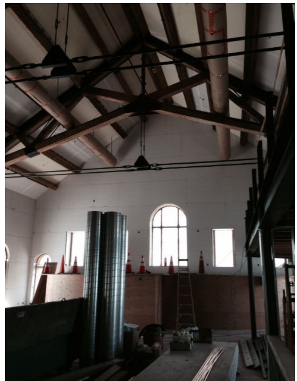
Work continues on the installation of the drywall in the 1921 main library portion of the building.
