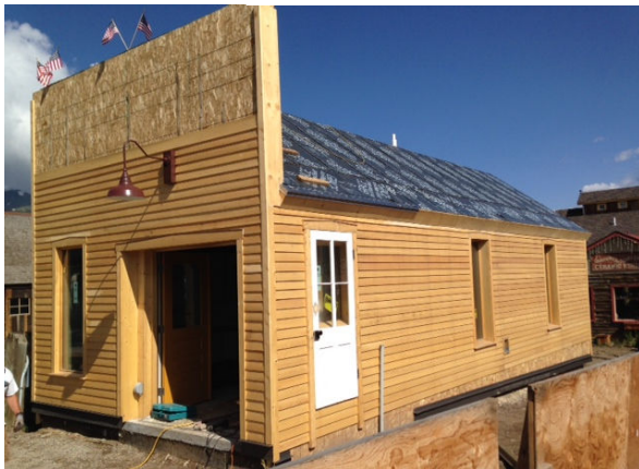
Siding is nearly completed on the Mikolitis barn. The false front was replicated from historic photos.
