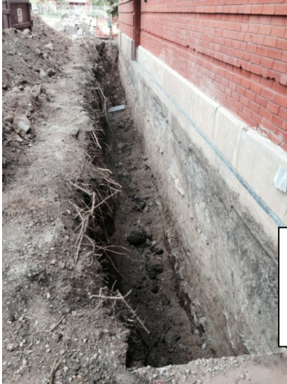
Excavation in front of the historic building in preparation of the installation of the storm drain system.
