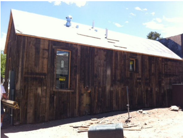
The historic siding was reinstalled on the west and north elevations of the Mikolitis barn.
