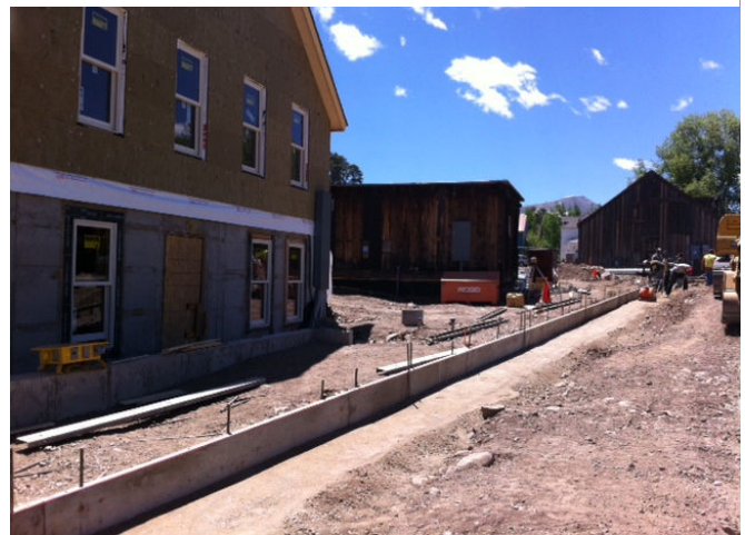
Forms for curb and gutter along the alley are set before the concrete is poured..
