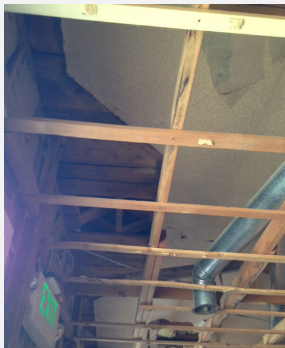
Looking up at the ceiling near the front door of the building. The shape of the white paper reveals the historic storefront dimensions.
