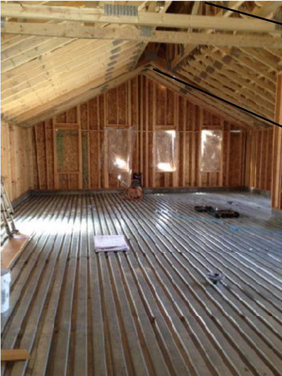
Above: Interior framing of Ceramics Studio and view looking into the monitor feature. The monitor allows natural light into the studio from above.
