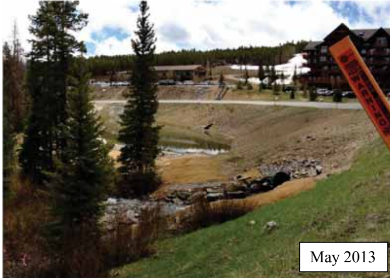
Photo C4b. Photopoint 2b, 2013. The restoration project included reconstruction of the culvert outlet structure and revegetation. The construction in the lower photo is for drainage from a new parking lot and hotel building. It is unrelated to the project.
