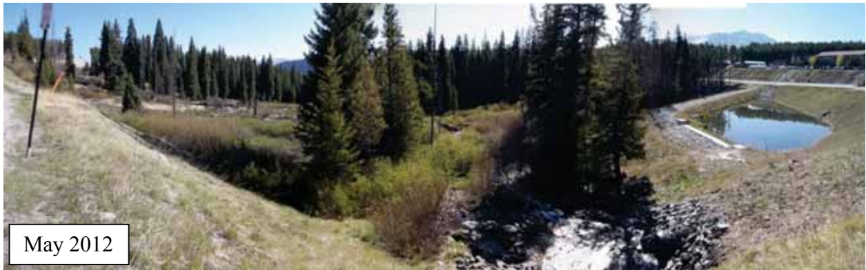
Photo C5a. Photopoint 3a, 2012. The photos show the development of treatments at the head of the Upper CG project area including reconstruction of the culvert outlet structure, a lateral distributary channel, and revegetation.
