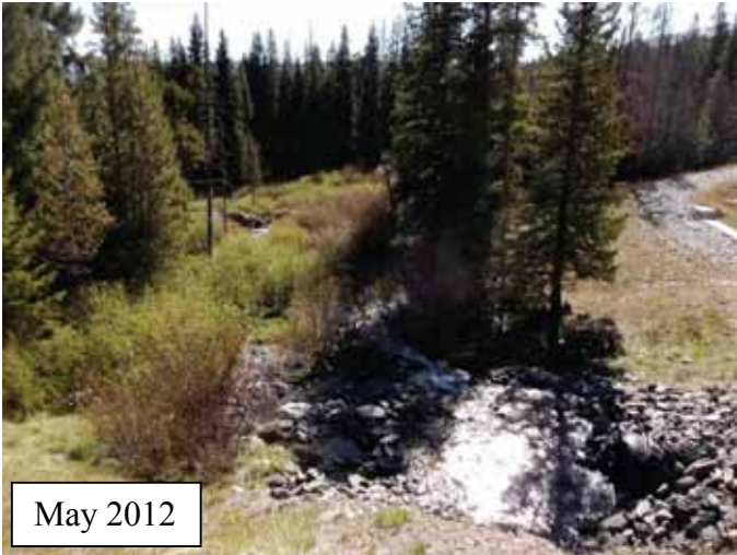
Photo C6a. Photopoint 3b, 2012. A closer view of the Boreas Creek culvert outlet.
