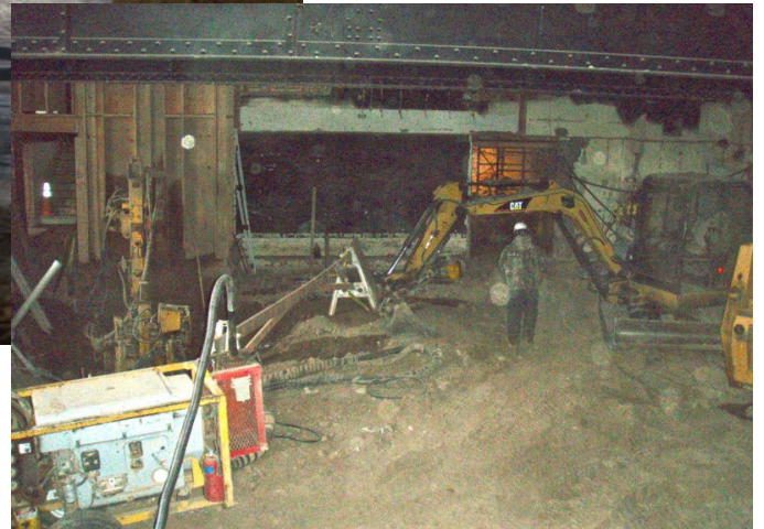
The removal of the existing basement concrete floors and embankment excavation in preparation of the new multipurpose room, restrooms, kitchen, coffee shop and movie theatre.
