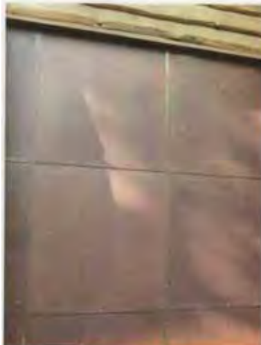
Rusted Metal Siding Sample
