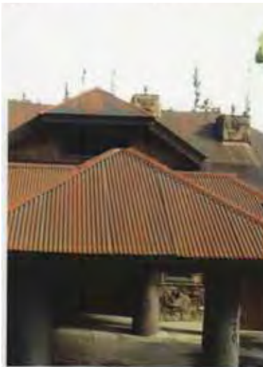
Rusted Cortin Roofing Sample
