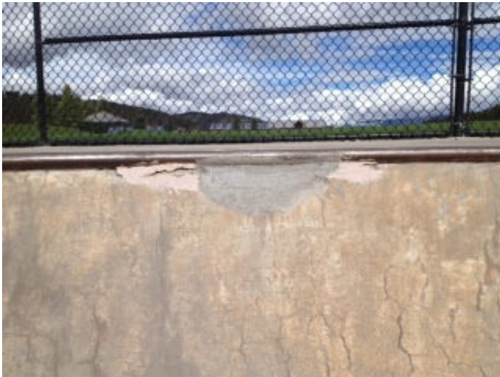
Problem area along coping in bowl that has been repeatedly patched
