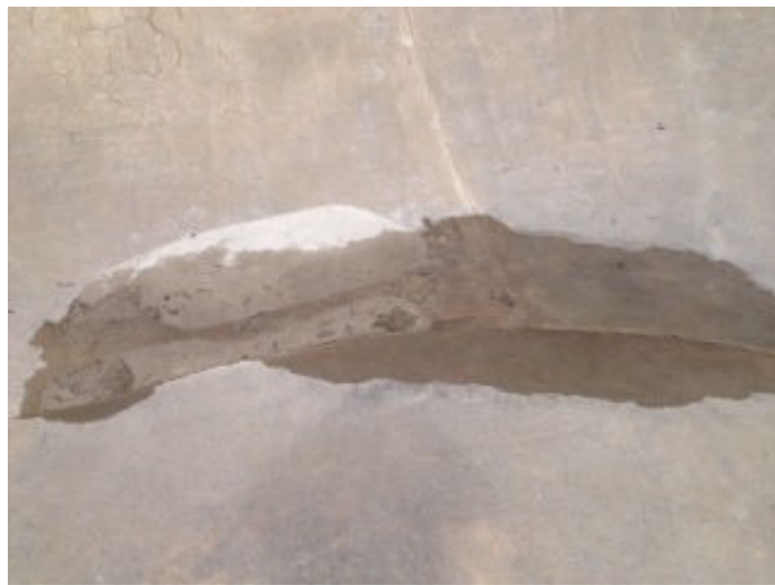
patched area in bottom of bowl and ineffective drainage
