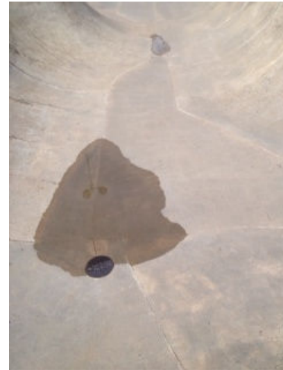
ineffective drain in bowl
