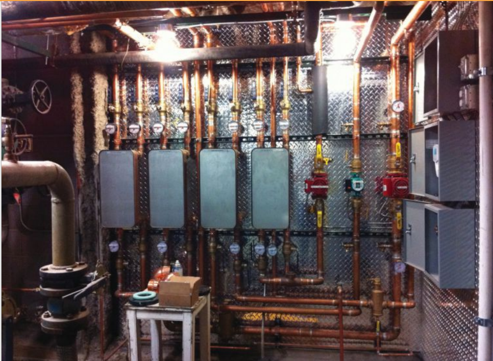
The team used larger heat exchangers on the project in order to improve efficiency. “On the incoming water side from the town, we’re seeing cold water get boosted to within 10°F of whatever the solar tank temperature is,” system designer Bob Kingston notes.
