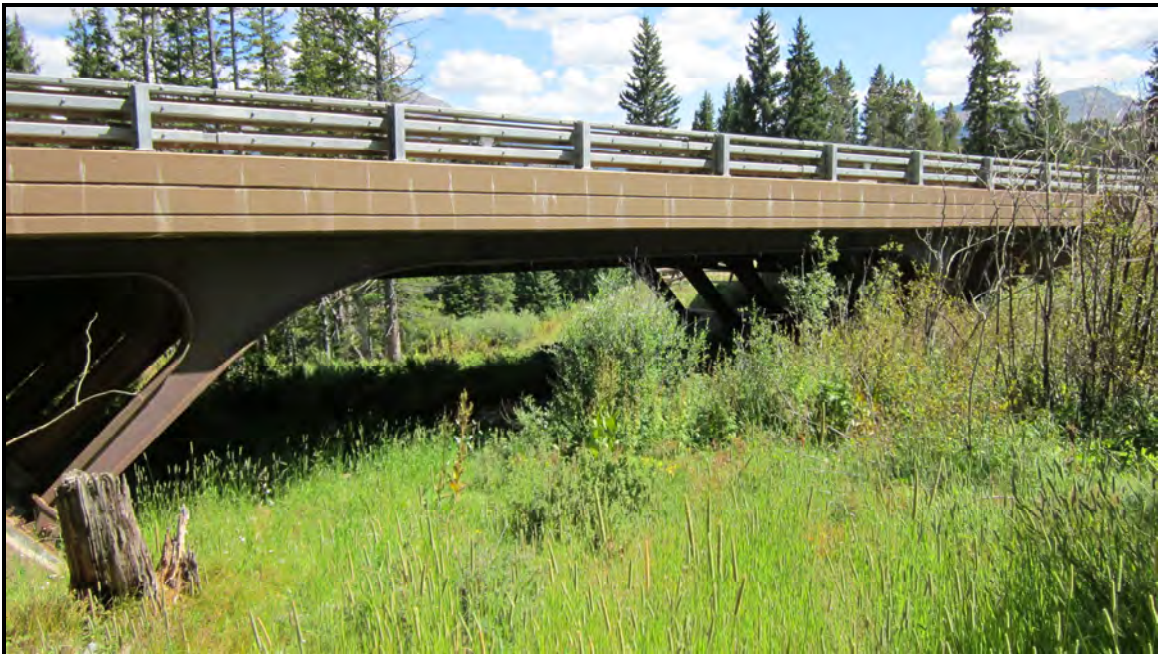
Photo 7. The realigned Ski Hill Road crosses over Bridge Creek via a bridge span rather than a culvert allowing much better hydrologic and migration connectivity between CGP and wetland habitats upstream. The bridge is high enough that everything from aquatic organisms to moose can pass through the opening.
