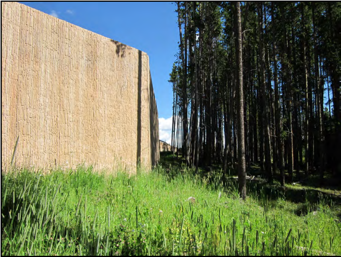
Photo 6. A concrete retaining wall constructed below Ski Hill Road and the Stables Lot in 2008 may influence local water distribution in addition to being a barrier to hydrologic connection and wildlife movement.
