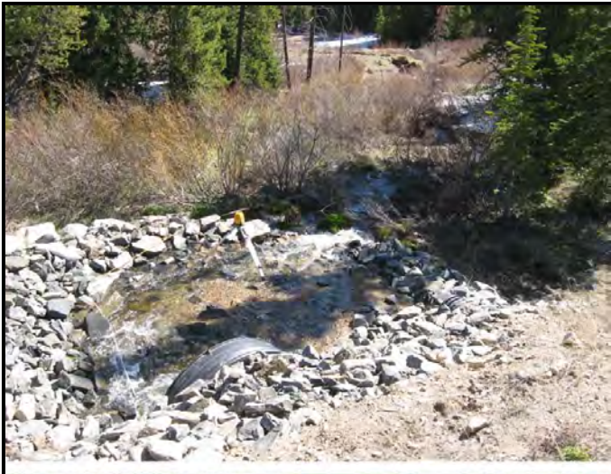
Photo 14. Boreas Creek enters Upper CG through this new 48" culvert. Water and sediment discharge from the Peak 8 watershed are concentrated by drainage systems above to this single channel. These photos show the culvert and the rock diversion structure below it. The upper photo is from early June. The lower photo is from early August. The rock structure has eroded, an indication of high stream power associated with this channel.
