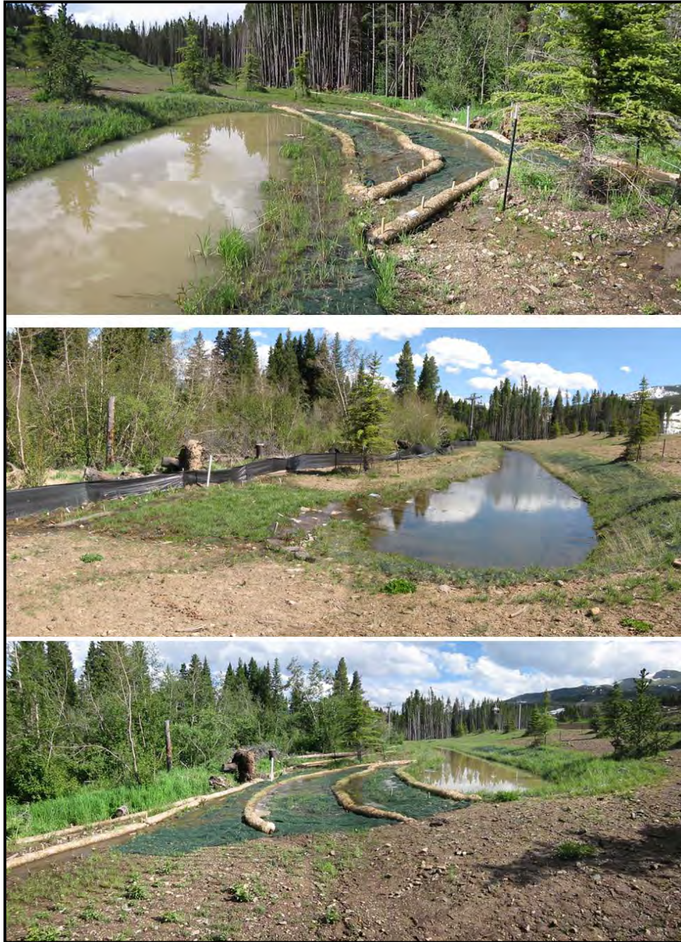
Photo 5. The new trench at the bottom of the Peak 7 drainage system is filled at its south end, and it spills at its north end (shown here). The upper photo is a view north of the outlet. The lower two show it looking south. The middle photo shows the outlet as it looked in May. The lower photo shows it in July, after a set of wattle check dams was installed.
