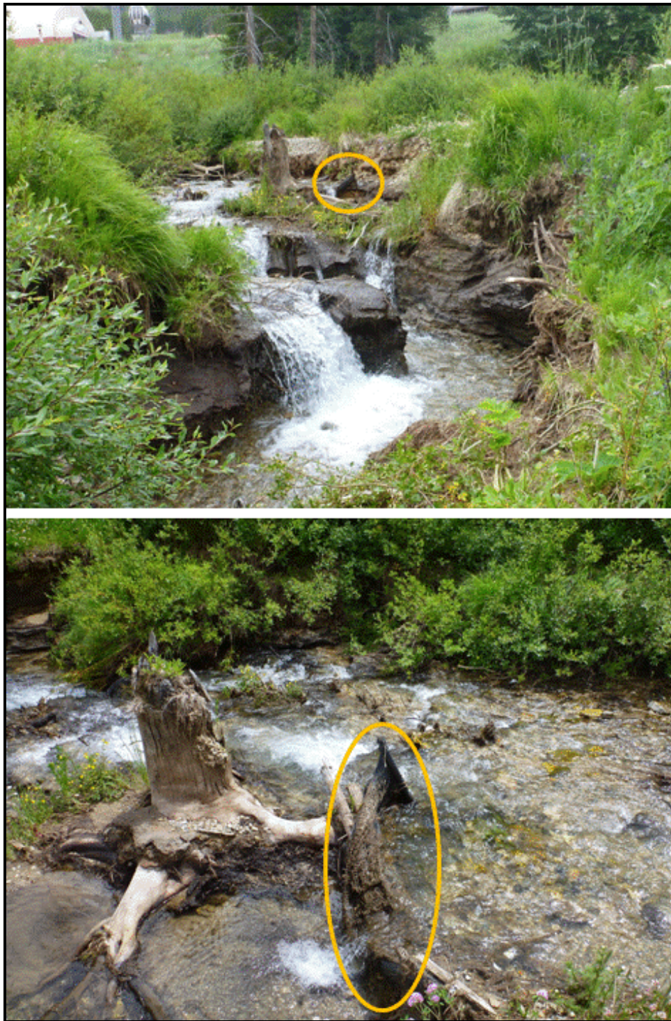
Photo 27. This photo gives a clearer view of the "exhumed" sediment fence (circled) within the enlarging Boreas Creek channel. The base of the fence and the base of the adjacent tree stump indicate the elevation of the streambed at the time the fence was installed. Since the time that fence was installed up to the time the dam broke, about three ft. of coarse sediment had filled the pond, effectively raising the ground surface by that height. Now, the creek is cutting through these sediments, and deeper, leaving the new ground surface "high and dry."
