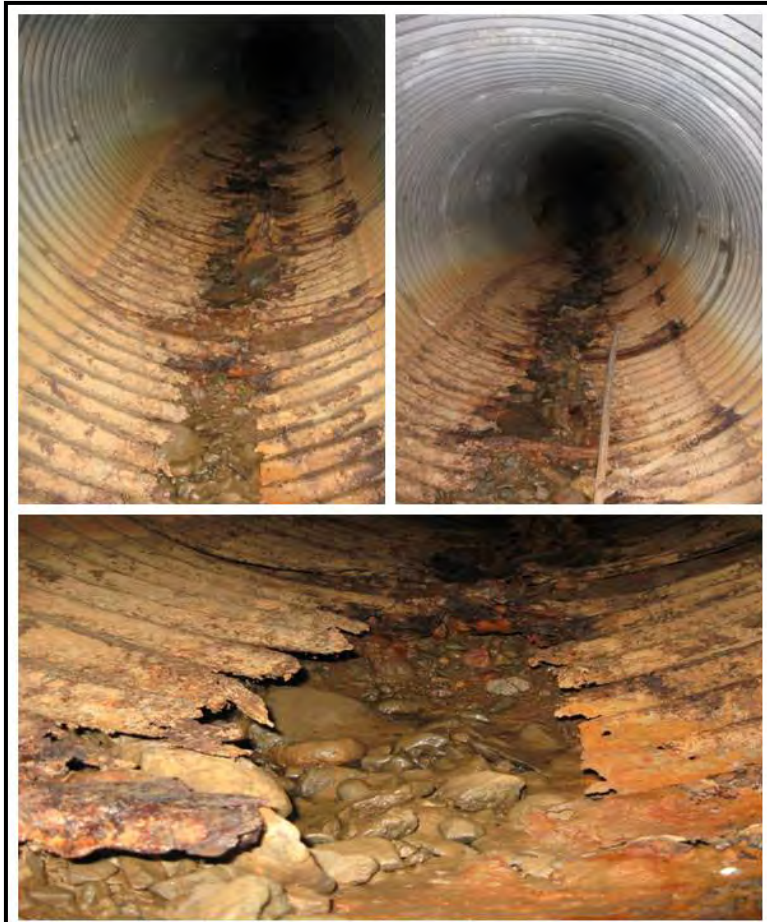
Photo 20. Photos from within the old Boreas Creek culvert (underneath Ski Hill Road) show that the bottom of this old pipe had completely rusted through. Some portion of Boreas Creek flows probably used to drain out of the pipe and into the ground while this old culvert was in use. A new culvert was installed recently, so any incidental spreading action of this old pipe is now no longer in play.
