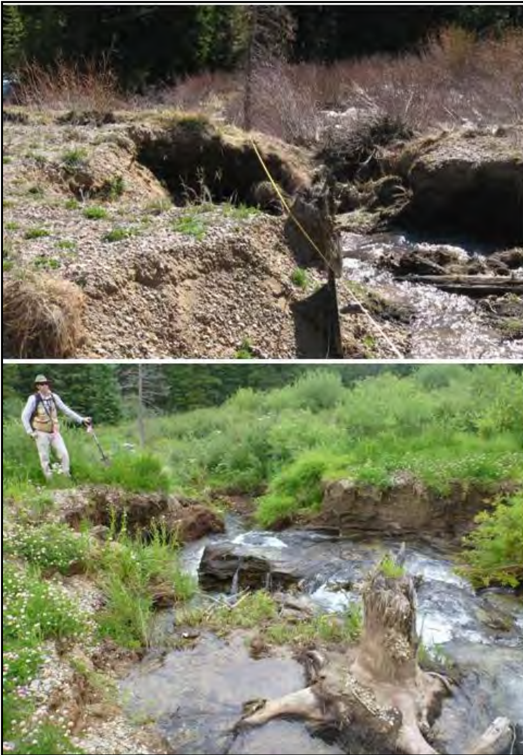
Photo 18. These photos show a view of the spreader pond dam taken from a point upstream (within the historic bed of the pond) in early June (upper photo) and mid-July (lower) of 2011. The dam had clearly begun to breach prior to this season, but the job was finished during July of 2011. Prior to this, the dam had functioned by impounding water and diverting much of the flow northward (left) to outlets on that side of the pond. Now, water flows directly through this area in one single, larger channel. Notice that the volume of the pond (in front of the dam) is completely filled with allochthonous sediment. In the upper photo notice the black piece of sediment fence at the bottom middle of the picture which is buried in sediment. The creek is now down-cutting through this sediment and even further down into ancient sediments that were below the level of the bottom of the pond.
