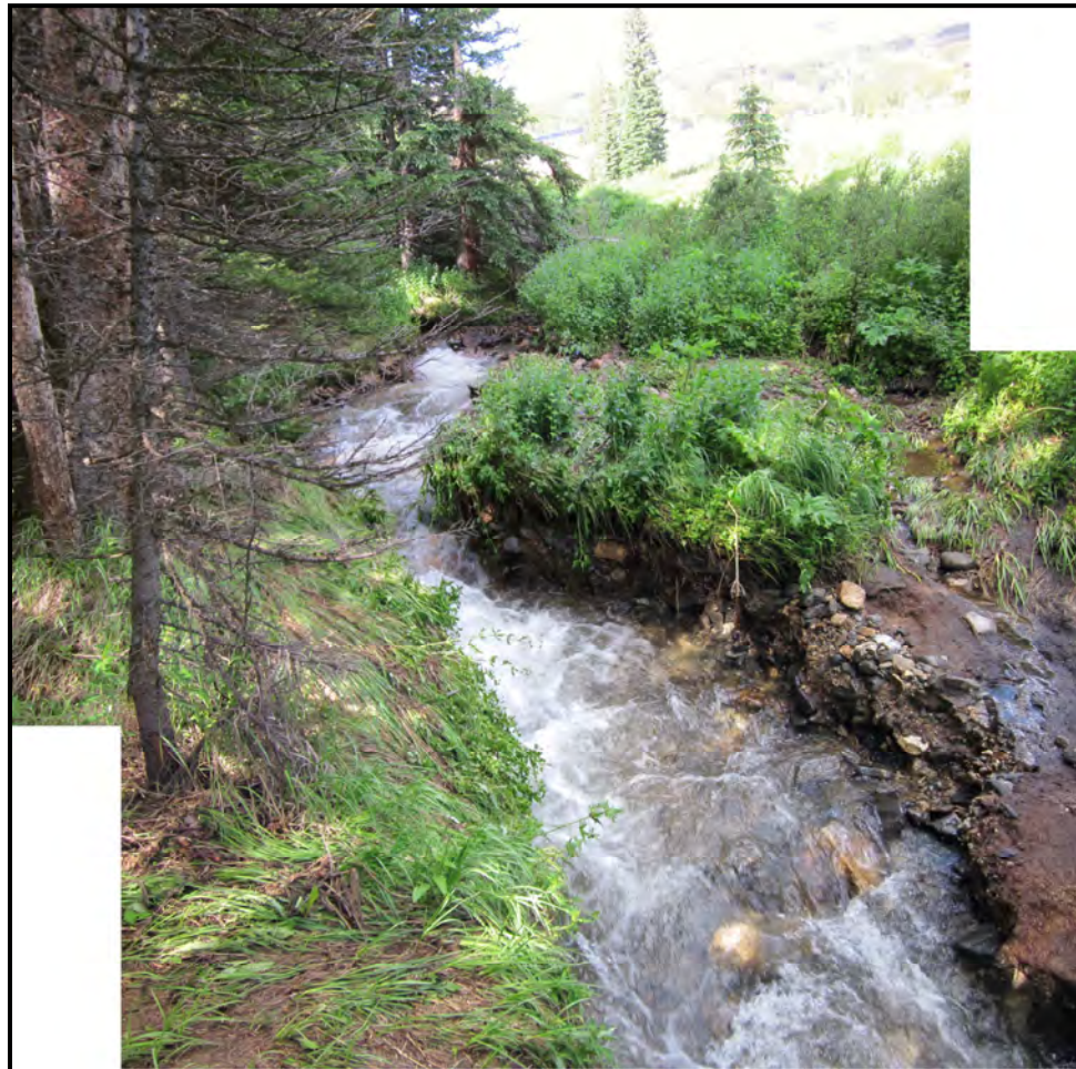
Photo 23. Channel incision occurred on segments of on Boreas Creek throughout the length of Upper CG in 2011. This photo shows a segment about 600 ft. downstream of the culvert which down-cut about 1.0-1.5 ft.
