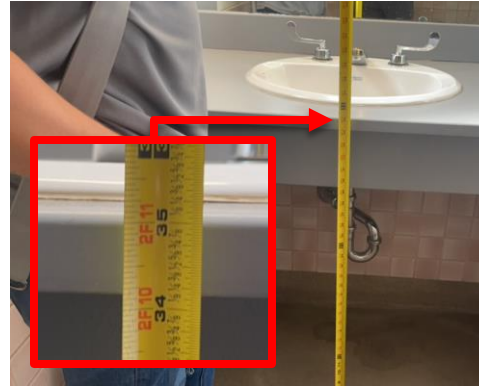
Measurement of lavatory sink is too high. 34" maximum.
