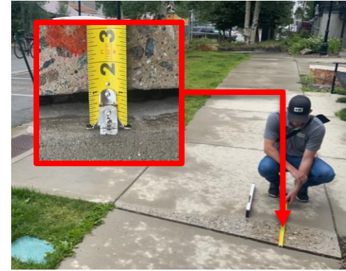
Measurement of gap in surface is too wide. 0.5" maximum.
