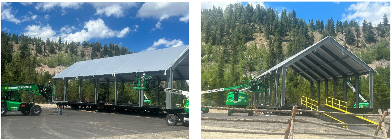
The temporary sprung structure framing is in place and the fabric roof and walls are currently being installed.
