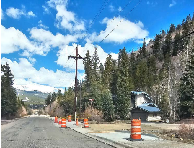
Boreas Pass Road looking west. Milling operations remove the top 2” of asphalt which is then replaced providing a new roadway surface.
