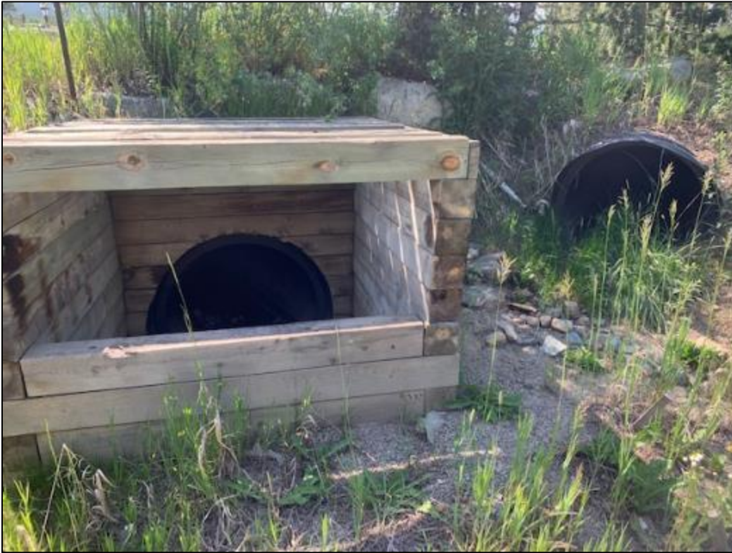
Photo 9 - Close up view of the outlet box showing no signs of flow, looking south (July 20, 2021)
