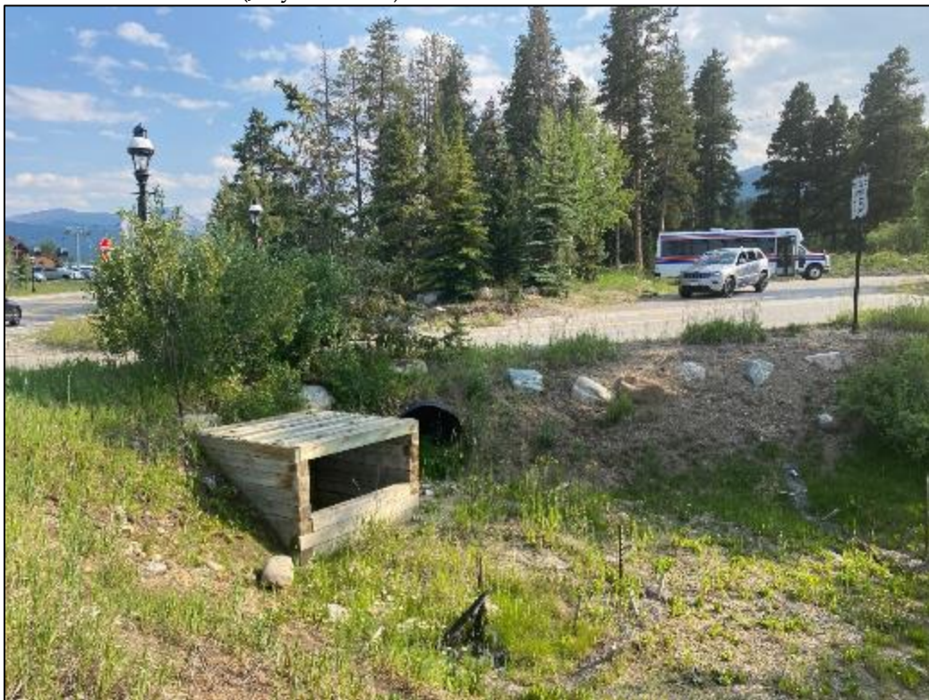
Photo 8 - Looking south at the culvert (black plastic) outlet under Woods Drive, with wooden outlet box to the stormwater system (July 19, 2021)
