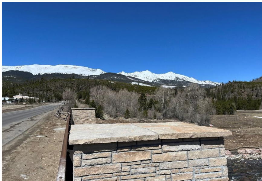
The stone caps at the top of the bridge columns were finished this week. The dirt shoulders and areas in the background of the picture will be graded and revegetated in the coming weeks.
