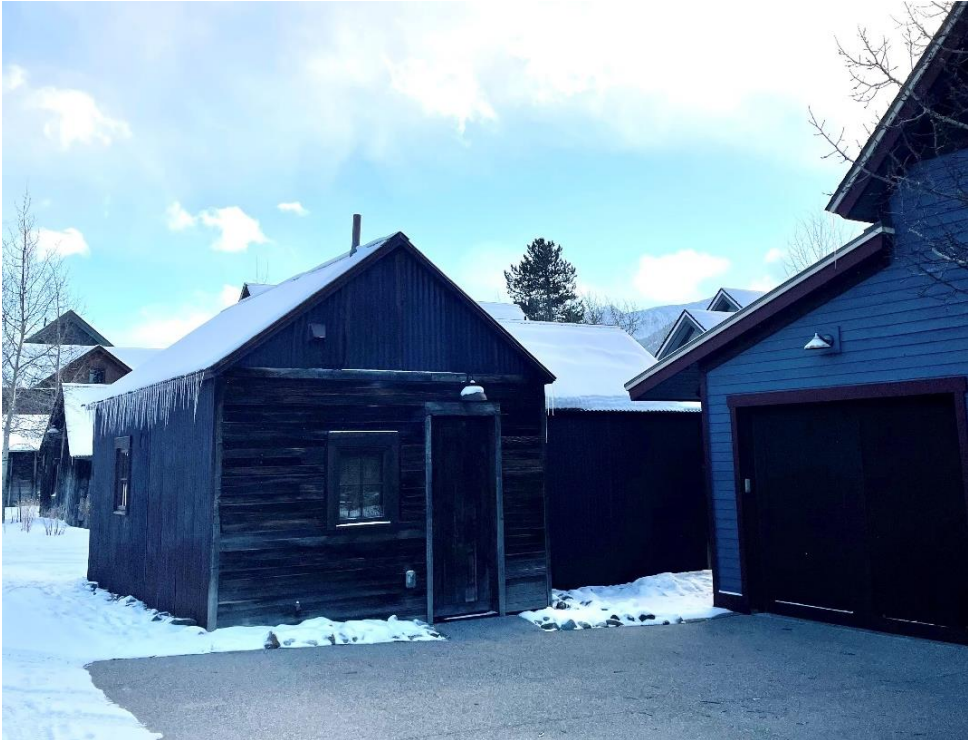
An example of a historic secondary structure with rusted metal siding located within the roof gable. Located across Lincoln Avenue on the Harris St. Alley.
