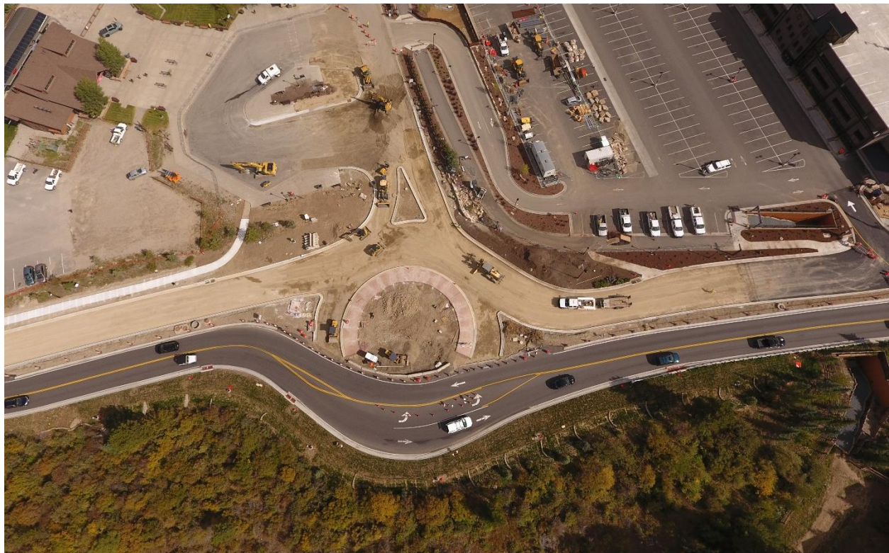
Most of the center concrete apron has been completed and the shape of the roundabout can be seen with the center circle in the middle and splitter islands at the ends.
