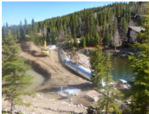
View of 96" diameter by-pass pipe.
