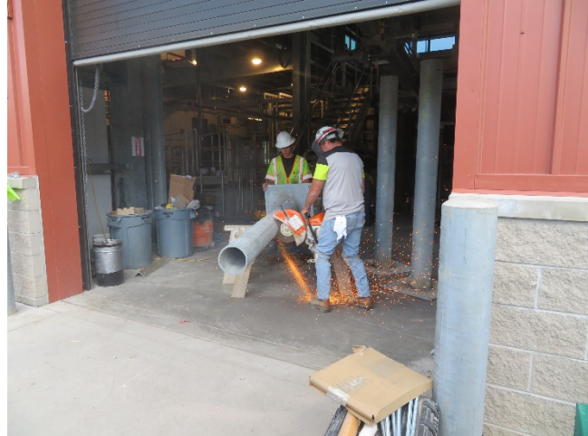
08/12/2020 – Residuals Container Bollards
