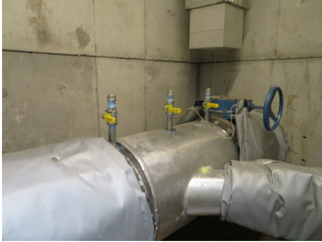
8/24/2020 - Blend Vault Future Chemical Injection Ports
