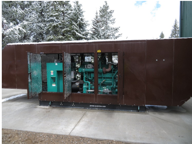
06/09/2020 – Raw Water Pump Station Emergency Generator.
