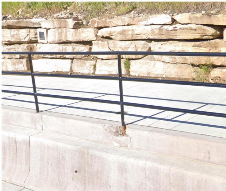
The photo above shows an example of a damaged portion of the retaining wall.
