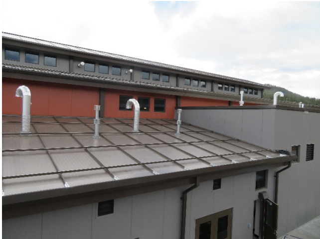
06/24/2020 – MTB Snow Retention System
