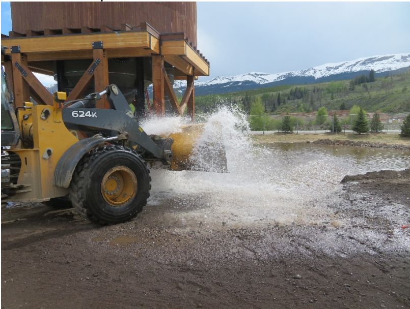
Raw Water Pipeline Flush 06/03/2020
