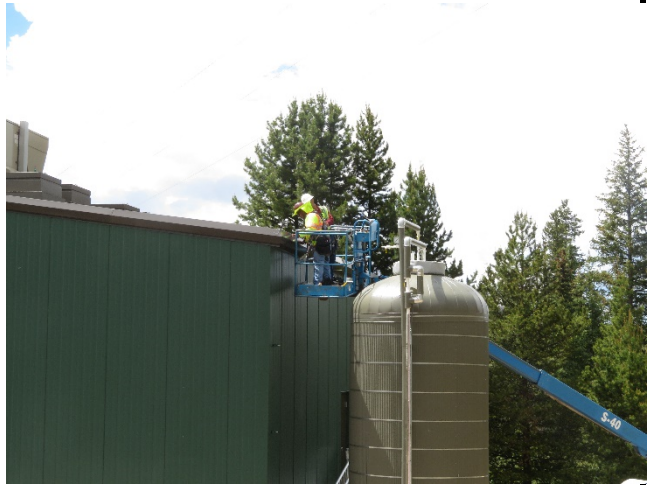
06/22/2020 – RWPS East Gutter
