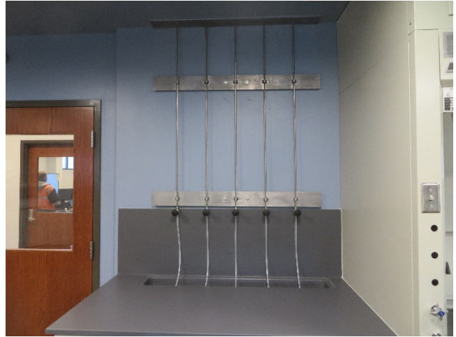
06/03/2020 – Laboratory Sample Piping
