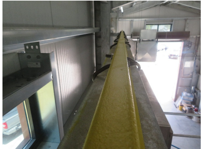
06/01/2020 – Bridge Crane Rail
