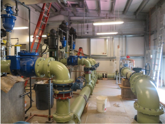
05/06/2020 – Raw Water Pump Station Painted Process Piping
