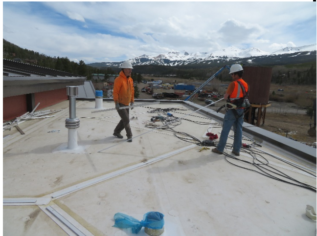
05/13/2020 – TPO Roof Heat Trace
