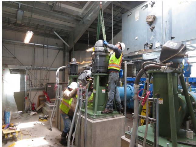
04/16/2020 – FWPS Vertical Turbine Pump Motor
