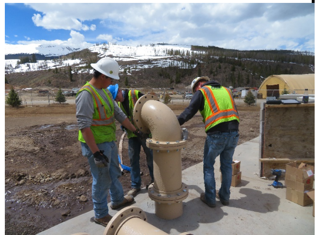
04/30/2020 – Backwash Waste Basin Gooseneck Vents
