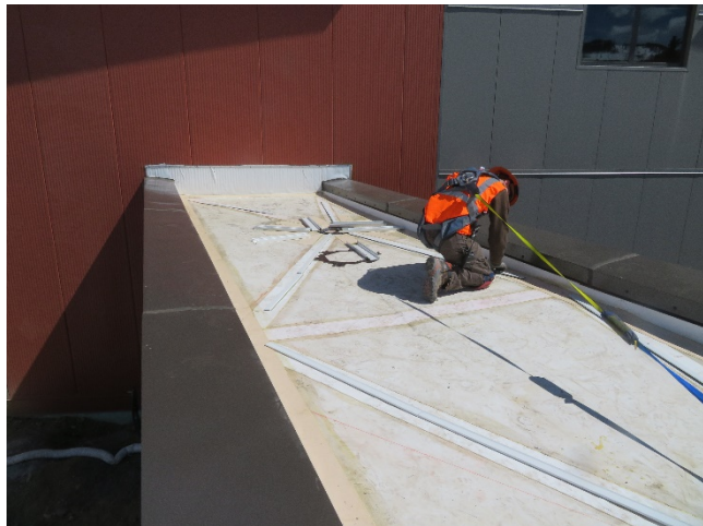
04/28/2020 – Covered Walkway Heat Trace
