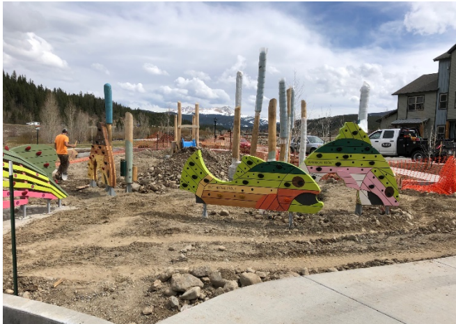
Custom play features, including “fish climbers”, being installed in the tots play area.
