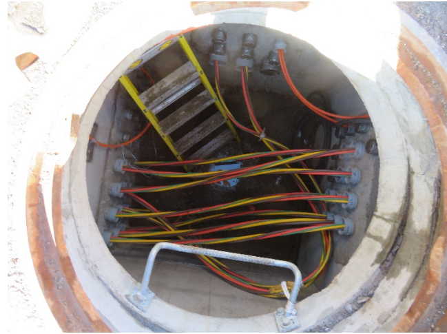
04/10/2020 - Electrical Hand Hole
