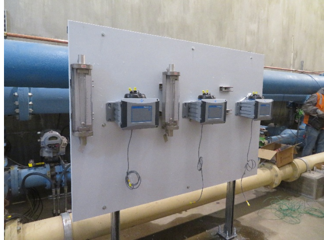
04/15/2020 – Filter Pipe Gallery Turbidimeters Instrument Panel
