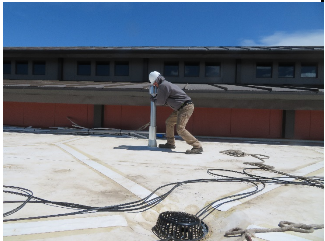
04/28/2020 – Unit heater Exhaust Pipe
