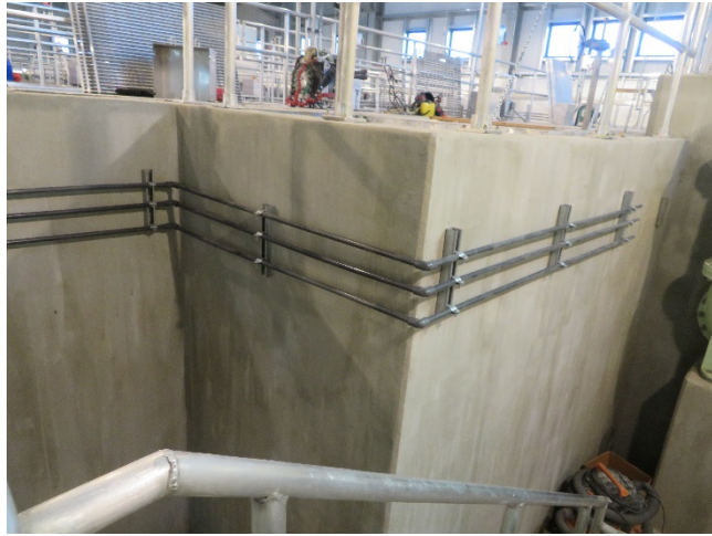
4/28/2020 - MTB Sample Piping
