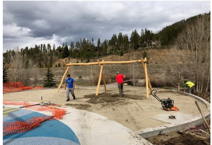
Log swings being installed which will include two standard swings, one infant swing, and one ADA swing.
