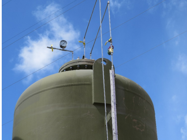
4/23/2020 - RWPS Surge Tank Instrumentation
