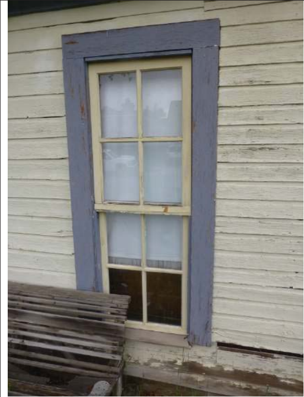
Figure 23: Recently installed sashes in Room 2 (casing appears original).
