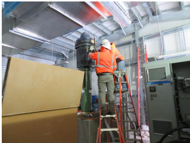
02/17/2020 – Raw Water Pump Station Vertical Turbine Pump Power Cables
