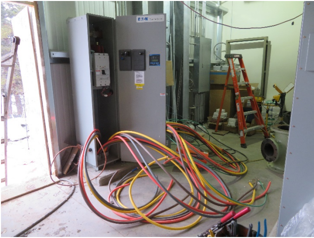
02/04/2020 – Raw Water Pump Station Main Breaker
