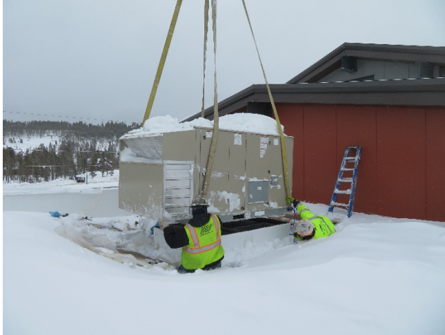
02/25/2020 - MTB MCC Room HVAC
