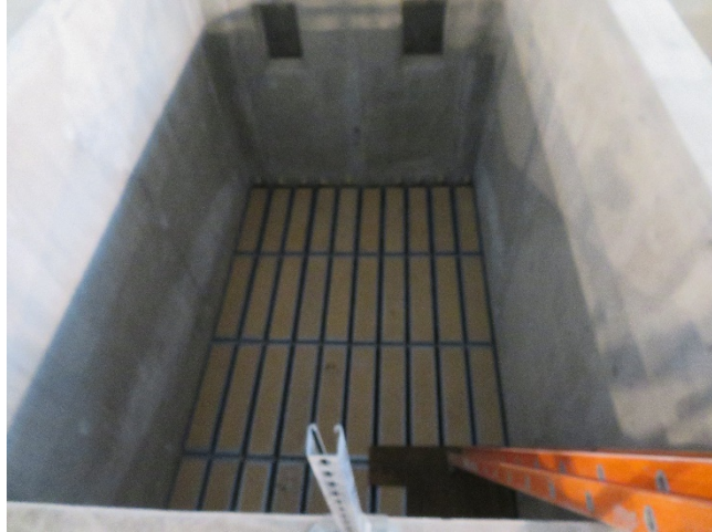
02/19/2020 - MTB Filter Underdrains
