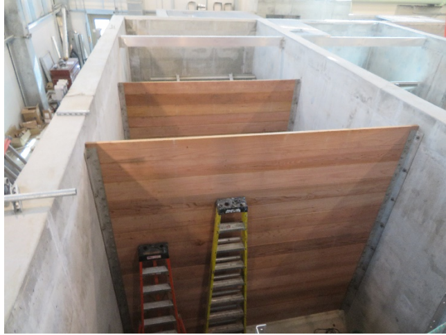
02/10/2020 - Flocculation Basin 1 Baffle Walls
