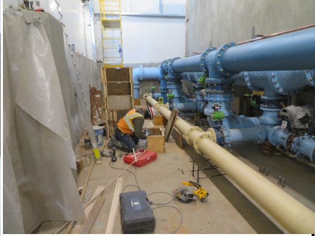
02/26/2020 – MTP Process Pipe Supports
