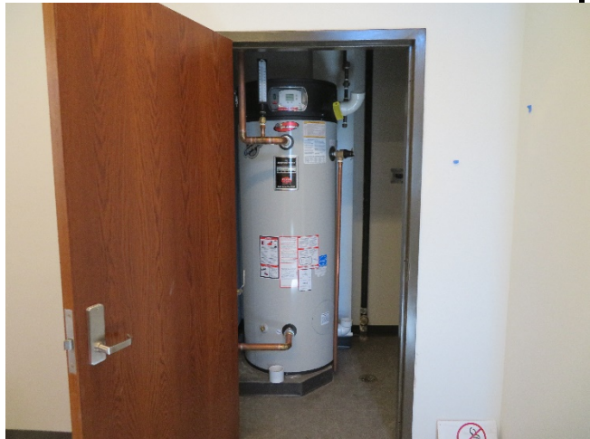
02/18/2020 – Administration Building Water Heater
