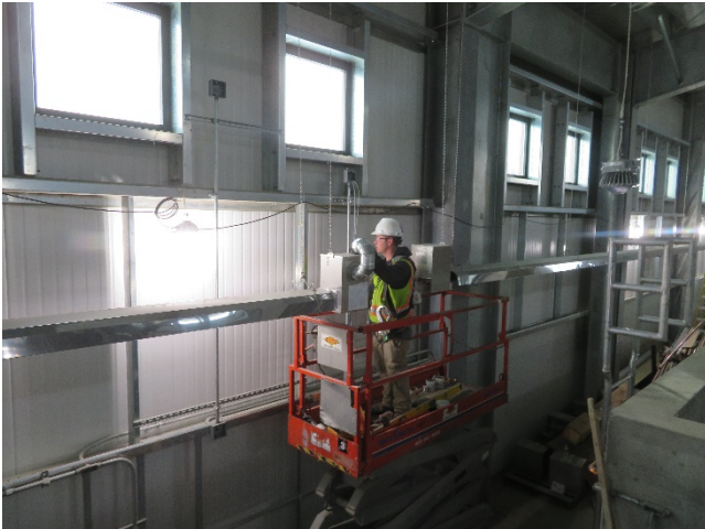
02/04/2020 – MTB Radiant Heat
