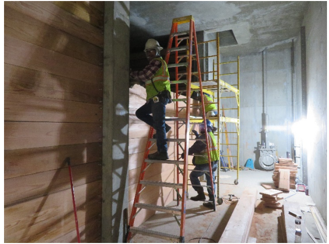
02/04/2020 – Clearwell Baffle Wall
