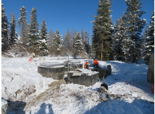
02/11/2020 – Raw Water Pump Station Valve Vault Heat Trace
