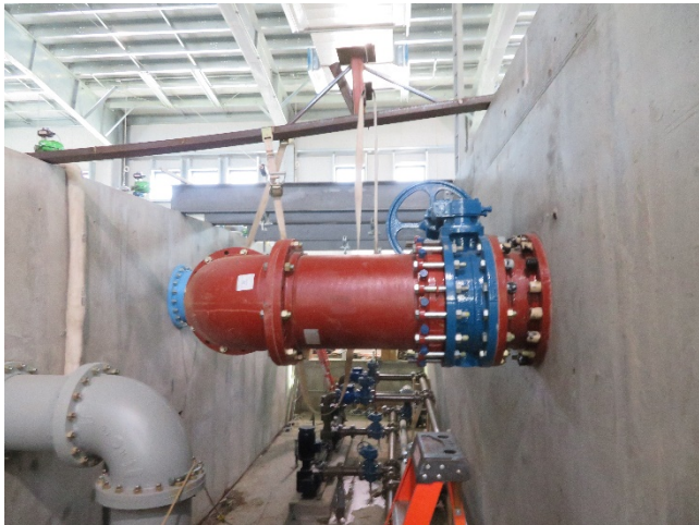
01/20/2020 – MTB Filter Influent Piping
