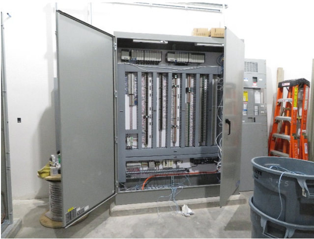
01/02/2020 – MTB PLC Cabinet
