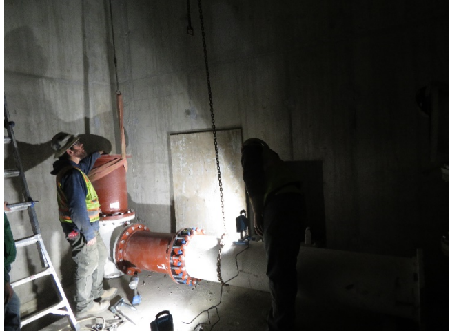
01/14/2020 – Raw Water Pump Station Wet Well Process Pipe
