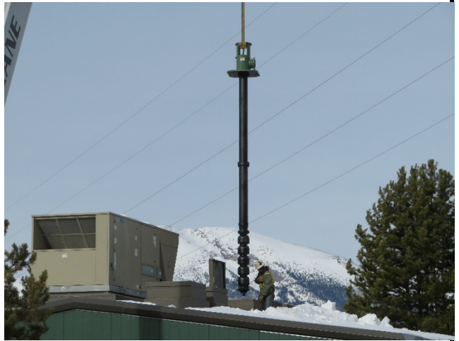
01/16/2020 – Raw Water Pump Station Vertical Turbine Pump
