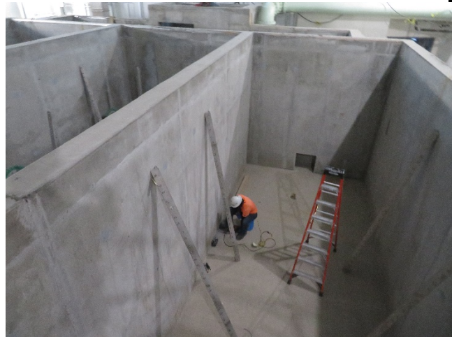
01/21/2020 – MTB Sedimentation Basin 3 Baffle Wall Angles
