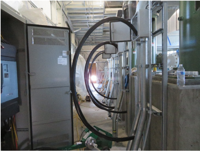
01/08/2020 – Finished Water Pump Station Vertical Turbine Pumps Power Cables
