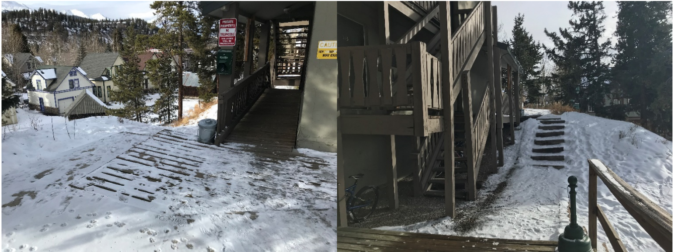
Figure 1&2: (North and South views) Existing south stairway, timber stairs and decking to be replaced.
