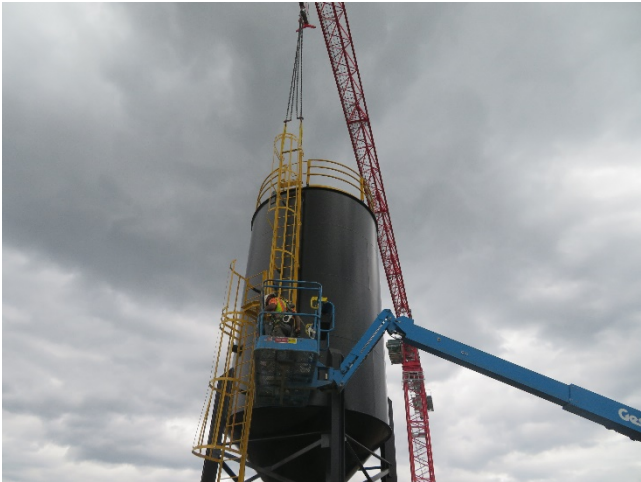
08/01/2019 Blend Tank Ladders
