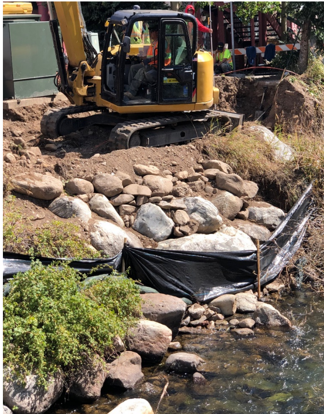
Excavation work being completed for a new retaining wall between the sidewalk and the river.
