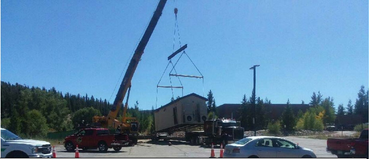
The central office or “hut” was delivered to the site near the County Justice Center.
