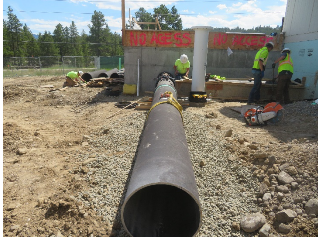
8/19/2019 - Clearwells Overflow Piping
