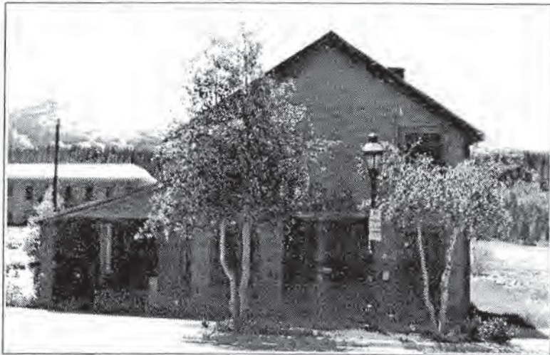
The same building as above, in which asphalt siding obscures the original materials. Original facade materials should be exposed and restored.
