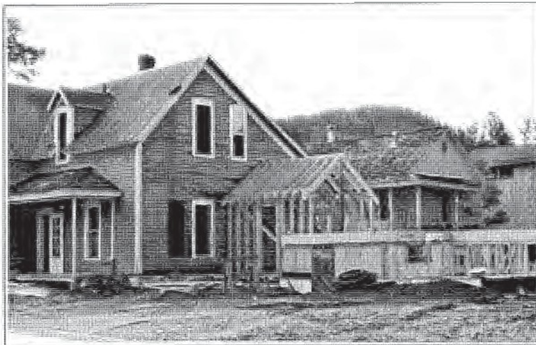
This rehabilitation project includes an addition that is separated from the original structure by a small connector, thus the historic scale and character are preserved.
