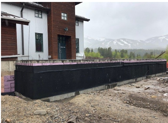
Foundation walls have been placed, waterproofed, and are now being backfilled. Plumbing will be roughed in and then the concrete slab will be placed.
