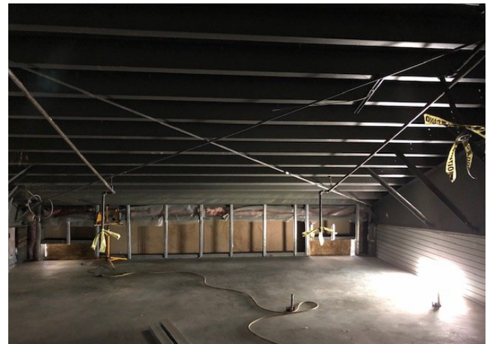
The concrete slab for office #2 (above Pro Shop) was recently placed and soon the walls will be framed and dry wall will be installed.
