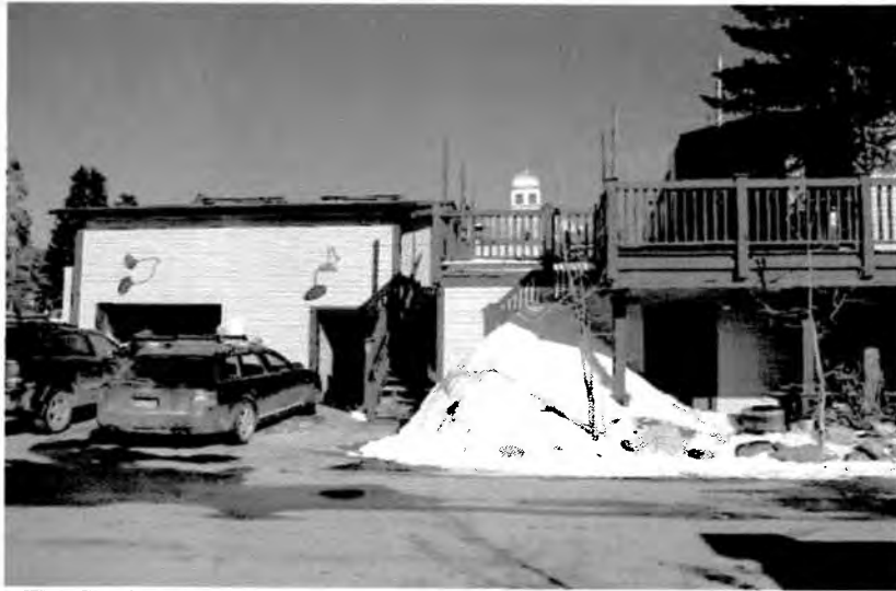
West Southwest Roof of Out Building at Rear of restaurant. An array of 5 collectors will be flush mounted below the skylights seen in this picture.
