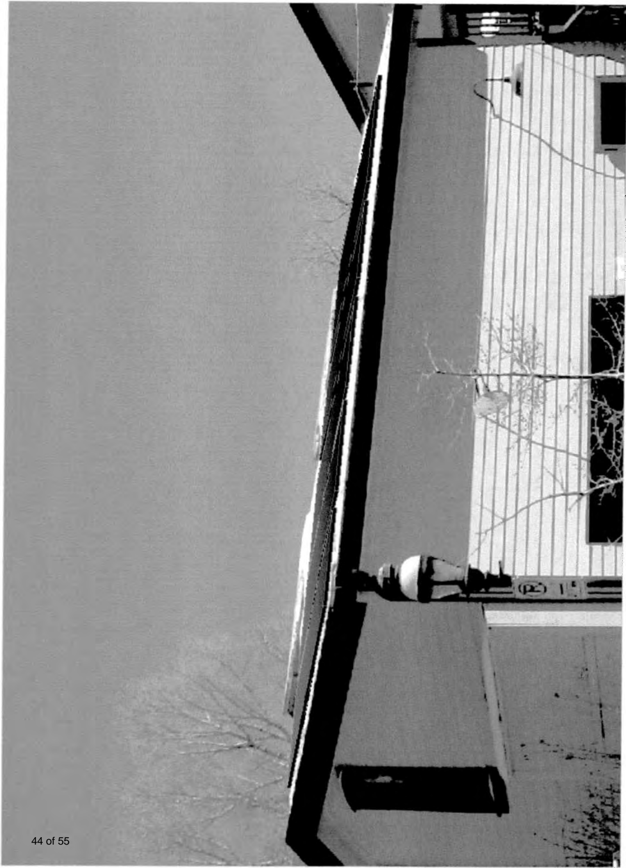
SALT CREEK SALOON -OUTBUILDING WITH (5) 4' X 8' FLUSH MOUNTED SOLAR COLLECTORS IN ARRAY
