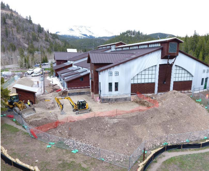
The excavation and backfill beneath the new foundations and slab has been completed at the northwest corner of the Ice Arena.
