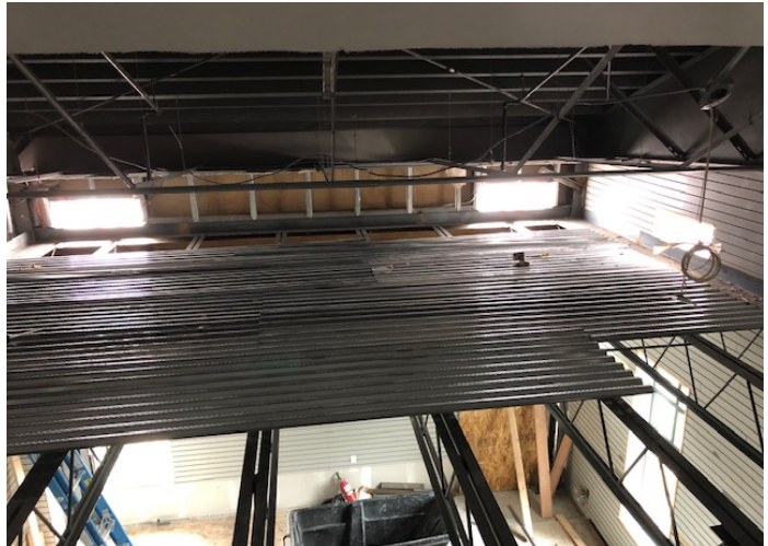
Steel columns, beams, and bar joists have been installed above the pro shop for one of the new offices. The existing ceiling at the top of the picture will be removed to create the office space.
