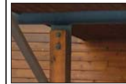
E14 EXPOSED BEAM POSTS RS DOUG FIR POSTS W/ PAINTED STL TUBE BEAMS
