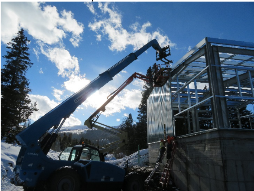
Raw Water Pump Station 11/07/2018
