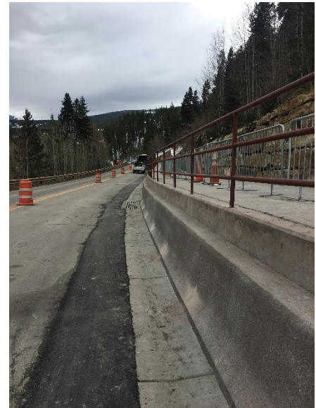
The replacement of the previous siloam stone retaining wall with the Type 7 Concrete Barrier shown above will increase roadway safety for vehicles.
