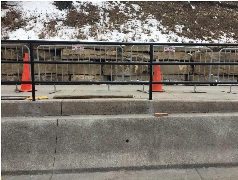
Final concrete finishing work will be completed in the next week for the retaining wall and barrier shown above, which will improve the surface and appearance of the colored concrete.
