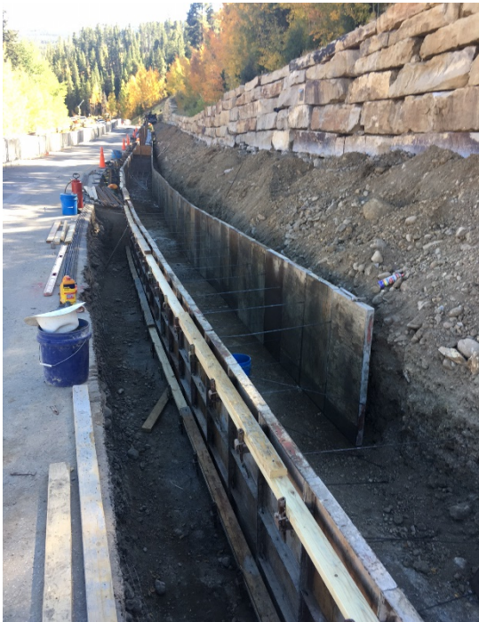
The existing wall was removed and the concrete footing for the new wall is being formed.
