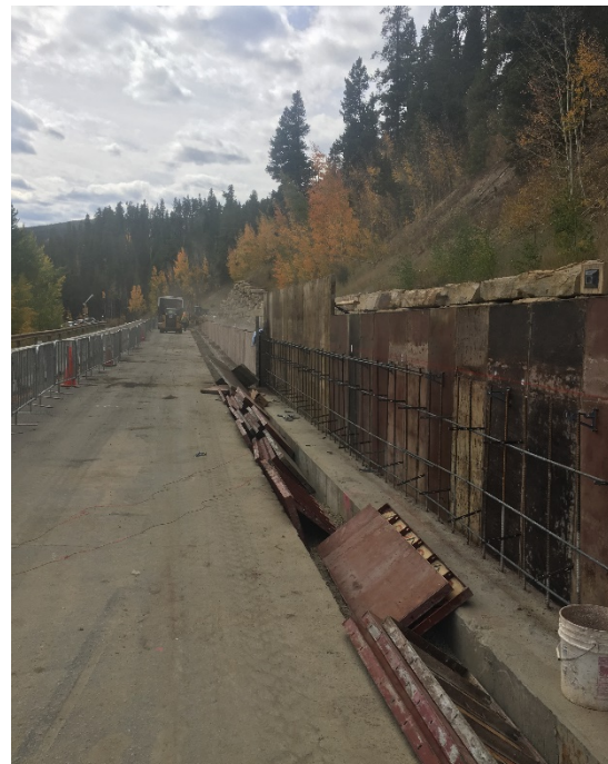
The new retaining wall is being formed and placed in the picture above.
