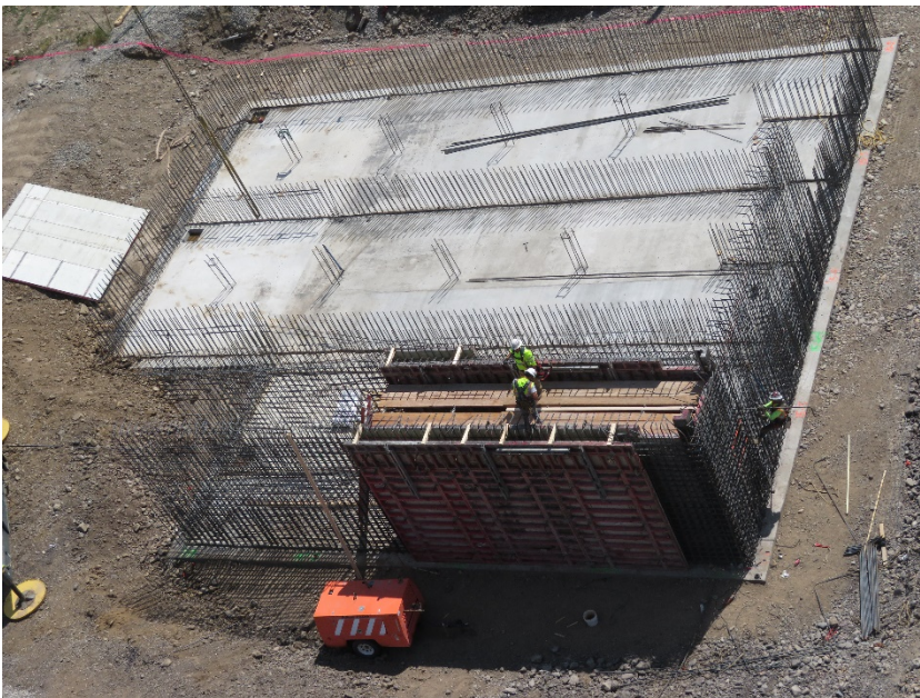
Finished Water Pump Station/Clearwell 08/10/2018
