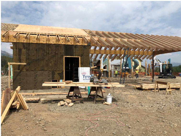
The picture above shows the roof framing being completed on the restroom/pavilion building.
