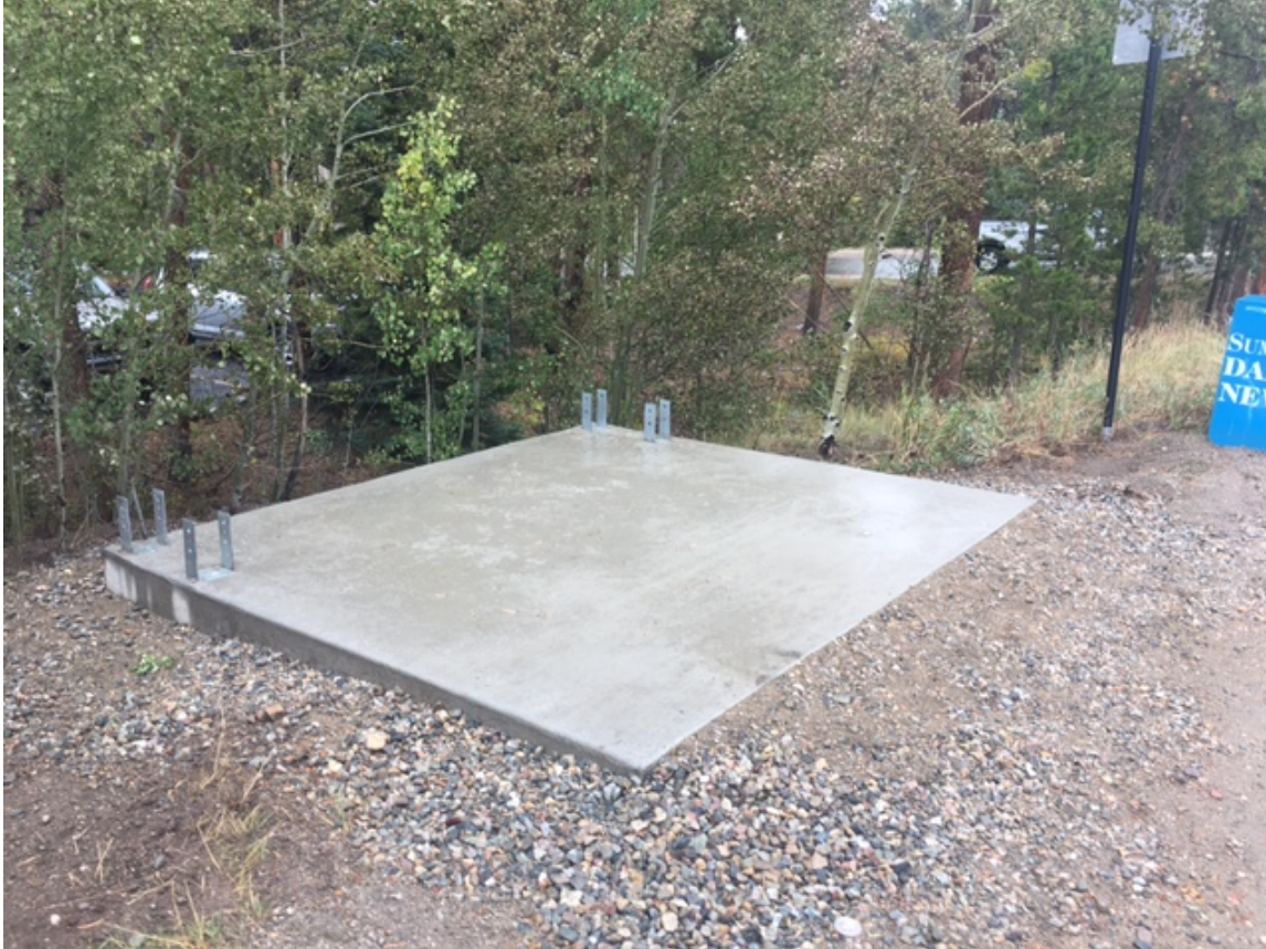
A concrete slab was recently constructed in preparation for the installation of the transit shelter.
